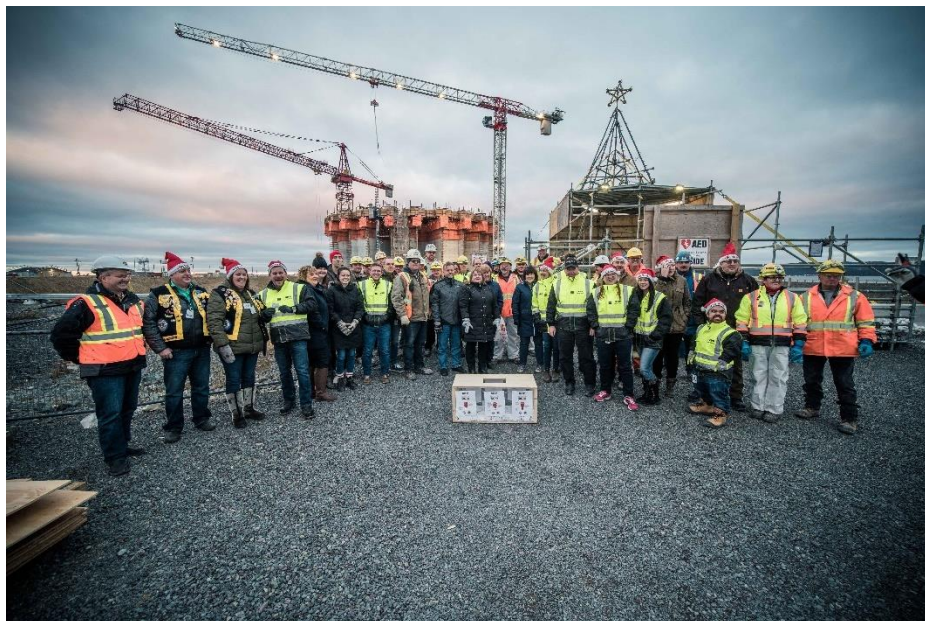
Employees at the West White Rose Project site in Argenteia collect and donate funds to the Zone 6 Region D Lion's Club. – December 2018
