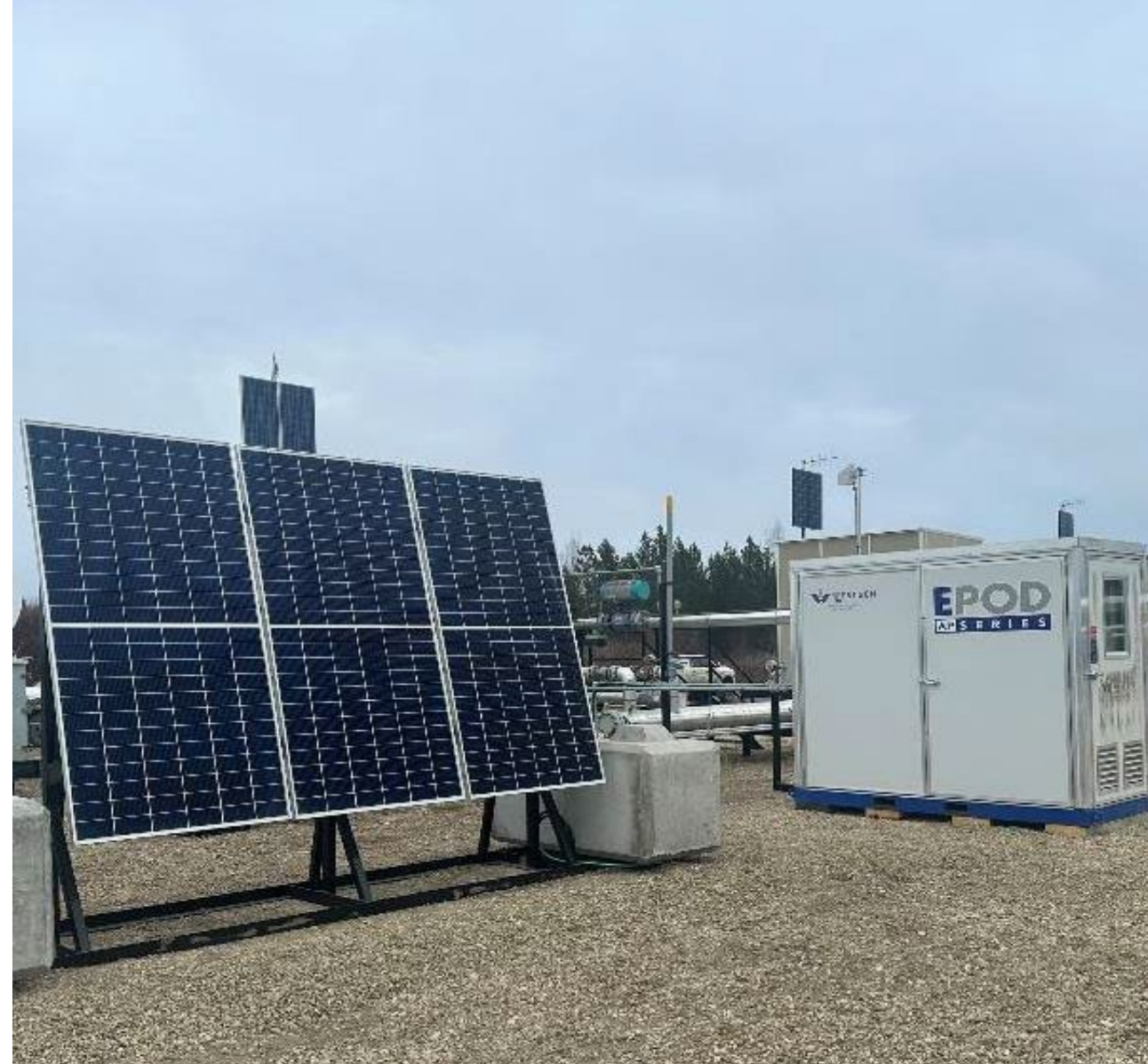
Instrument air package with solar panels as part of our Conventional GHG reduction program.
